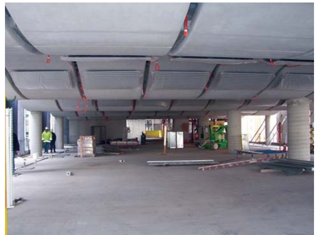
B. Plastic wrapped chilled ceiling panels and electrical services.
