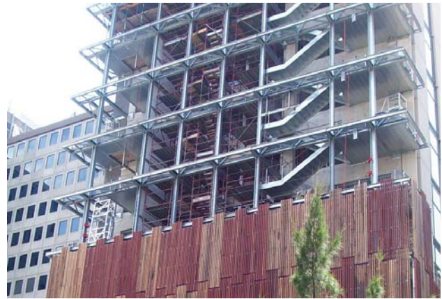
A. West internal access stair and pattern of active natural timber façade.
