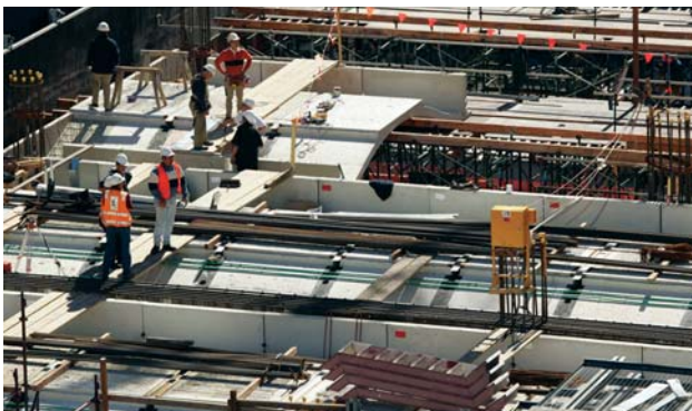
F. Positioning reinforcing steel and services. Green pipes are for cooling water supply for radiant chilled ceiling panels.
