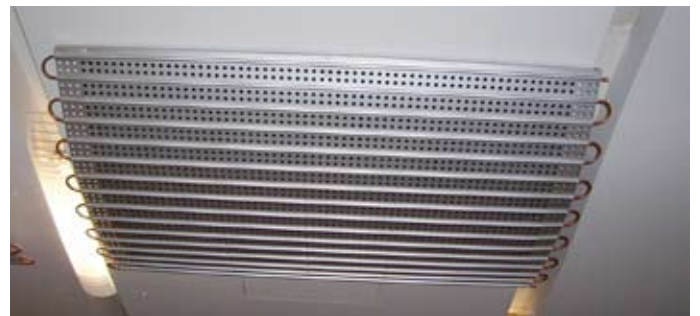
Figure 11. Chilled ceiling panel
