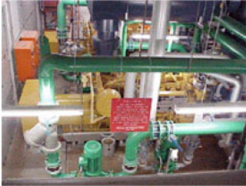
Figure 2. Example of a gas fired co-generation plant at Macquarie University, NSW. Source SEDA.
