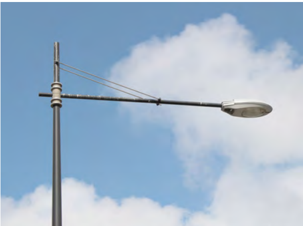
King Street light - short pole
