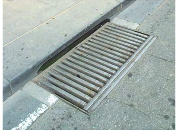
Drainage pit side entry with standard steel grate
