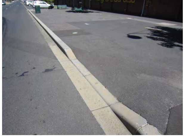
Crossing asphalt paving with no edging
