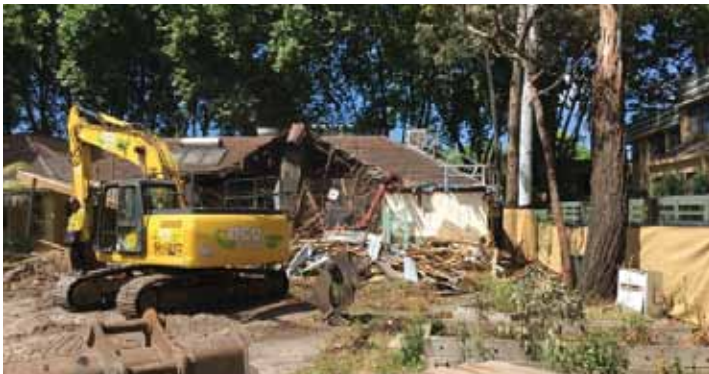
Above - demolition of the 70 year old 'American Colonial' style building which was built in 1939.
