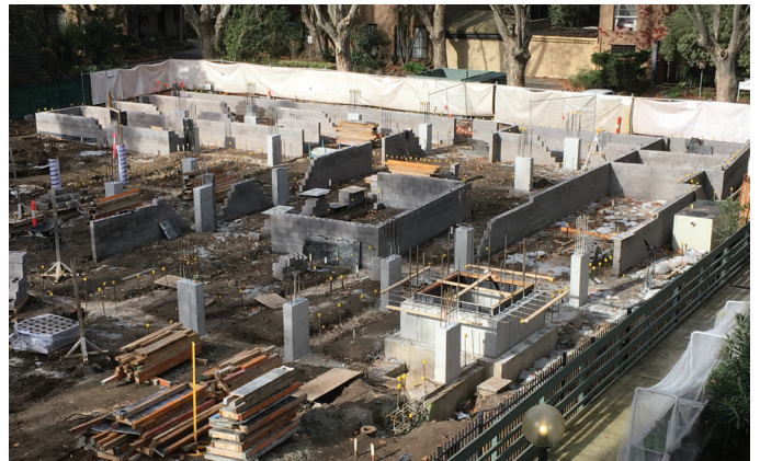
Construction works taking place from the rear of the site to the front.
