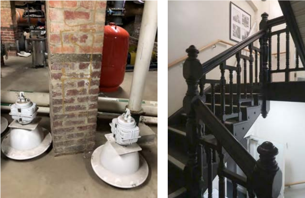
Figure 75 (a) Underpinning works below former men's pool; (b) southern staircase between ground floor and basement
