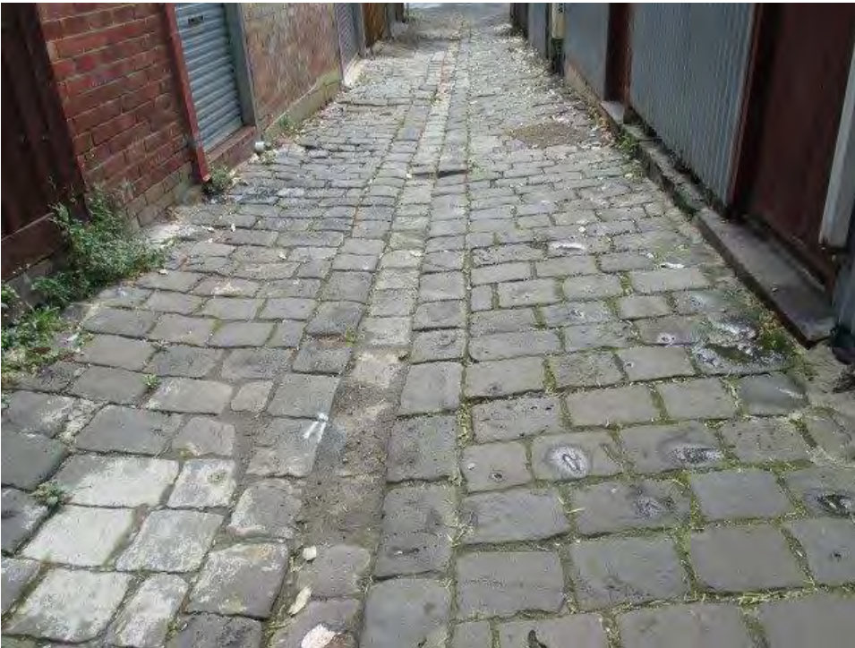
Figure 6: Munros Lane (Heritage Overlay Area) – Typical laneway requiring renewal prior to reconstruction
