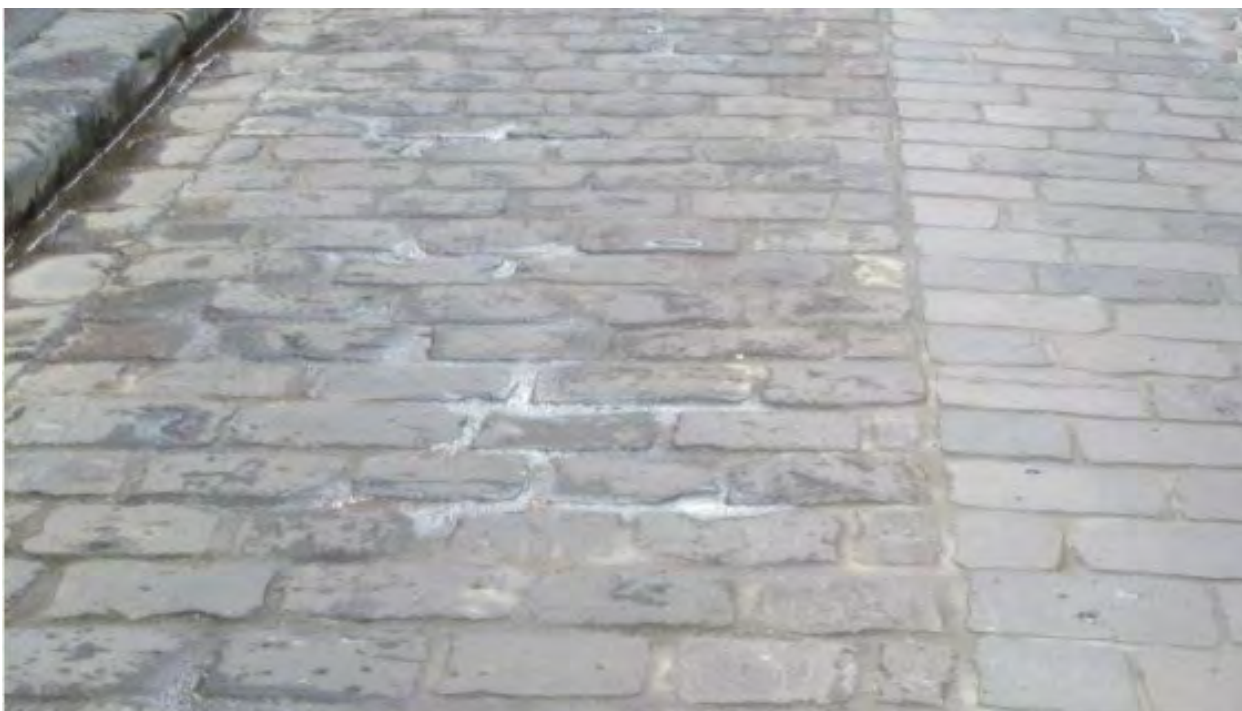
Figure 11: Little Errol St - picher laneway with half width pichers sawn (smooth) for Disability Discrimination Act access to The Arts House / North Melbourne Town Hall, built in 2013.
