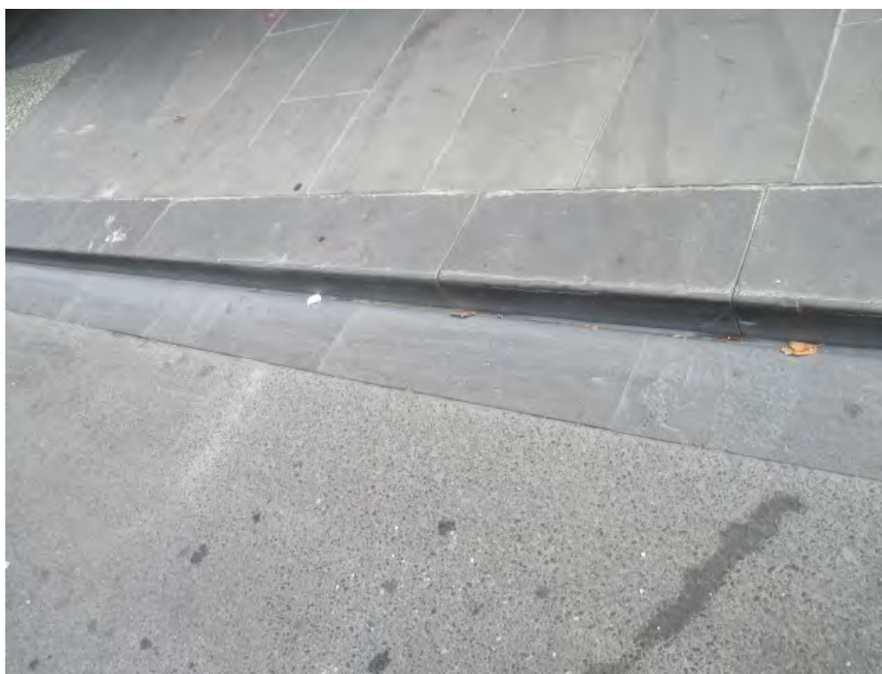
Figure 31: New sawn bluestone kerb and channel installed adjacent to sawn bluestone paving footpath
