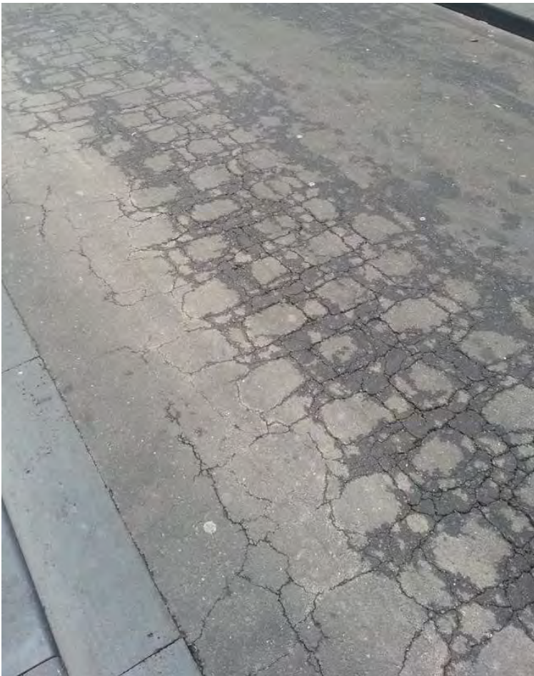
Figure 16: Westwood Place (prior to reconstruction) – Removed original pitchers overlaid with asphalt and reconstructed in asphalt pavement
