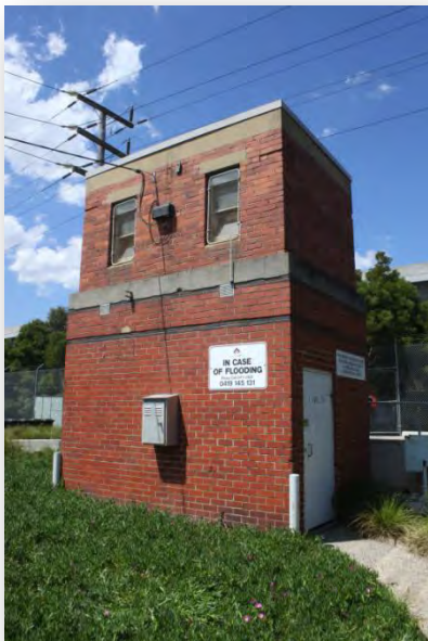
Figure 195 Stormwater pump house, off Stubbs Street, Moonee Ponds Creek
