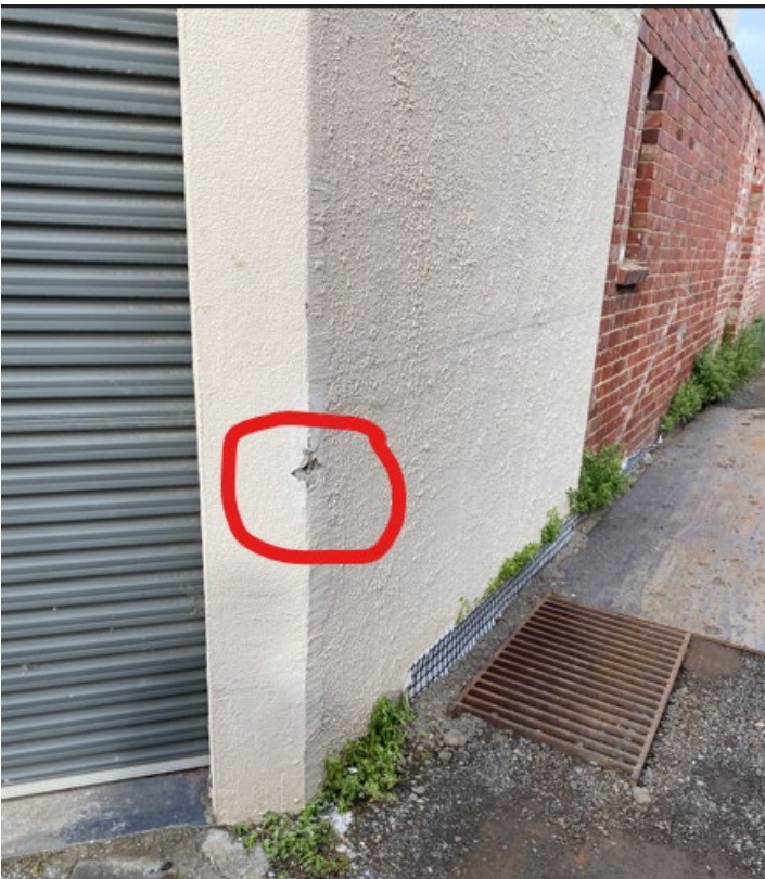
Photo 2 – Wall Damage in October 2023
