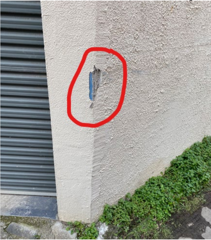
Photo 1 – Wall Damage in September 2023
