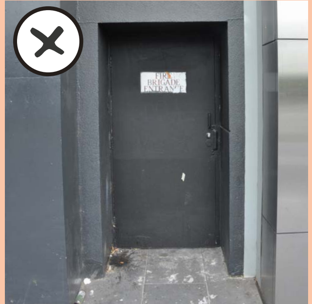
Alcoves and spaces related to service doors which result in entrapment space.
